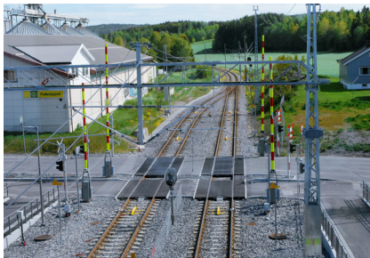
Helbomanlegg / Full barrier
